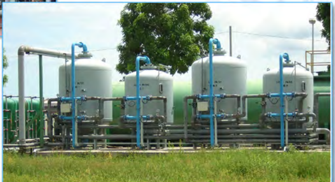
River Water Treatment System
