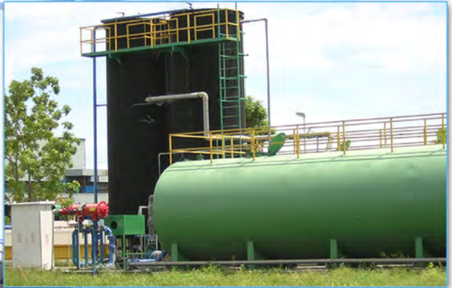
Tube Well Water Treatment System
