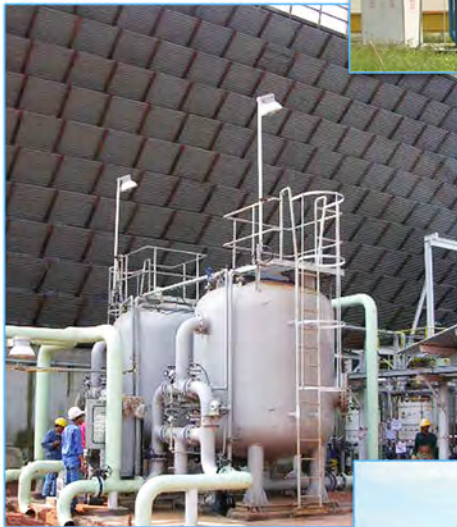
Cooling Tower Side Stream Filtration
